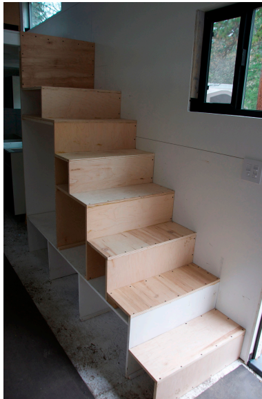
This set of stairs can easily be built by assembling custom cut plywood boxes strategically stacked on top of each other.
