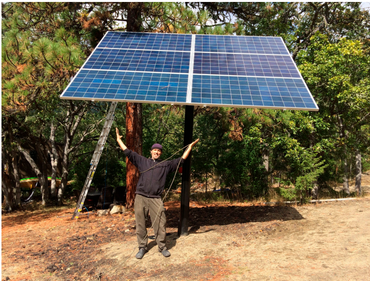
This image of Andrew shows the size of a 1.6 kWh solar array mounted on a pole. The pole is 8' deep and supported by tons of poured concrete to prevent any uplift in case of high winds.
