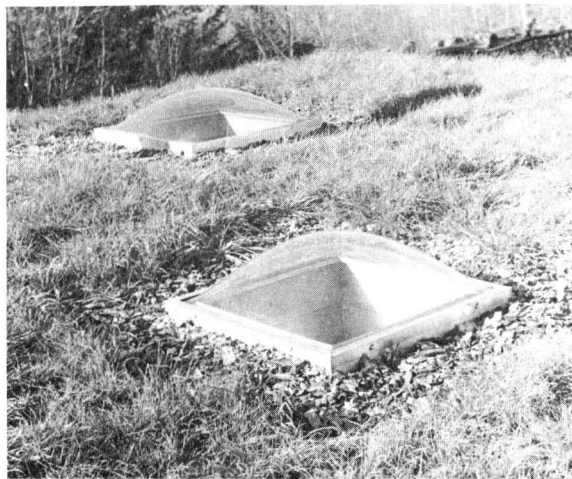
Fig. 99. Sand covered by woodchips provides the good drainage necessary to prevent leaks around skylights.
