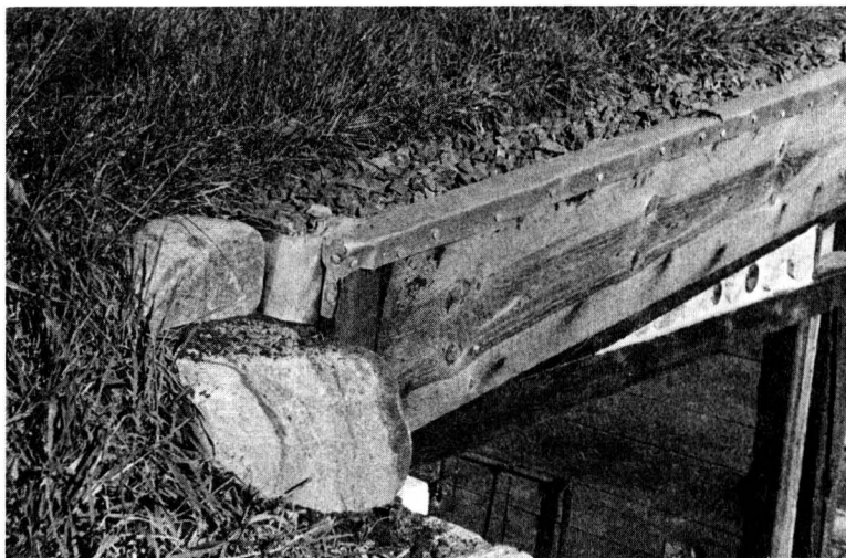
Fig. 100. Removing the sod within 5 inches of the retaining board and replacing it with a layer of sand covered by 6 inches of crushed stone improved the drainage and relieved the lateral pressure from the retaining board.
